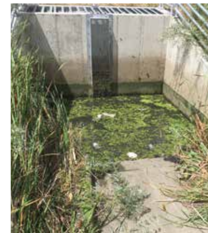
Stormwater management facilities can be permitted for routine maintenance with a Nationwide Permit 43, as long as wetland impacts are under 1/10 acre and returned to as-built conditions. Pond Outlet structure pictured above.
