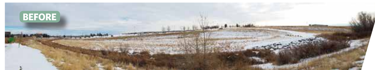
Dense and unfavorable vegetation along Windmill Creek within Regional Pond W-4 obstructed storm runoff conveyance prior to removing and recycling.
