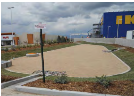
The sand filter basin on the IKEA site provides treatment for stormwater runoff
