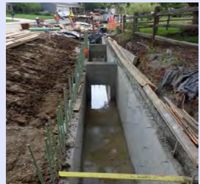
Additional storm sewer pipe to move water from the streets to the stormwater system
