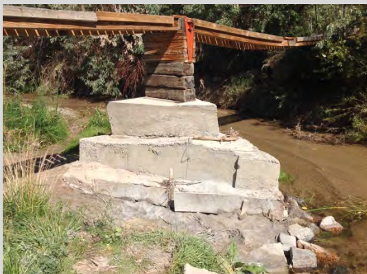
Un-permitted bridge crossing violated floodplain regulations
