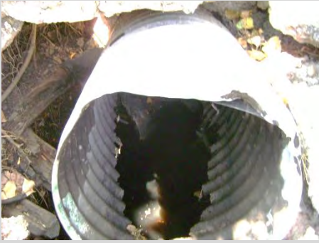
A corrugated metal pipe in critical condition
