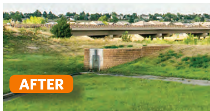
The Ladera Pond retrofit replaced boggy areas with healthy vegetation due to an improved outlet structure that allows the pond to drain and the bottom to dry out.
