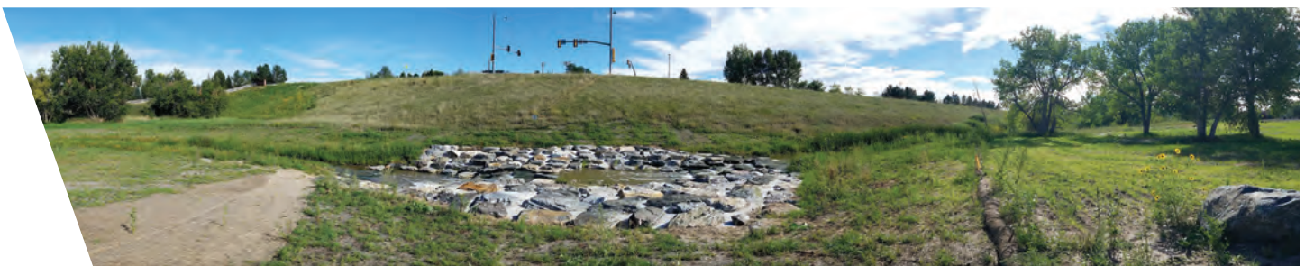
Construction of a grade control structure in Piney Creek to stabilize the stream, resolve the sediment supply problem, and mitigate localized flooding.
